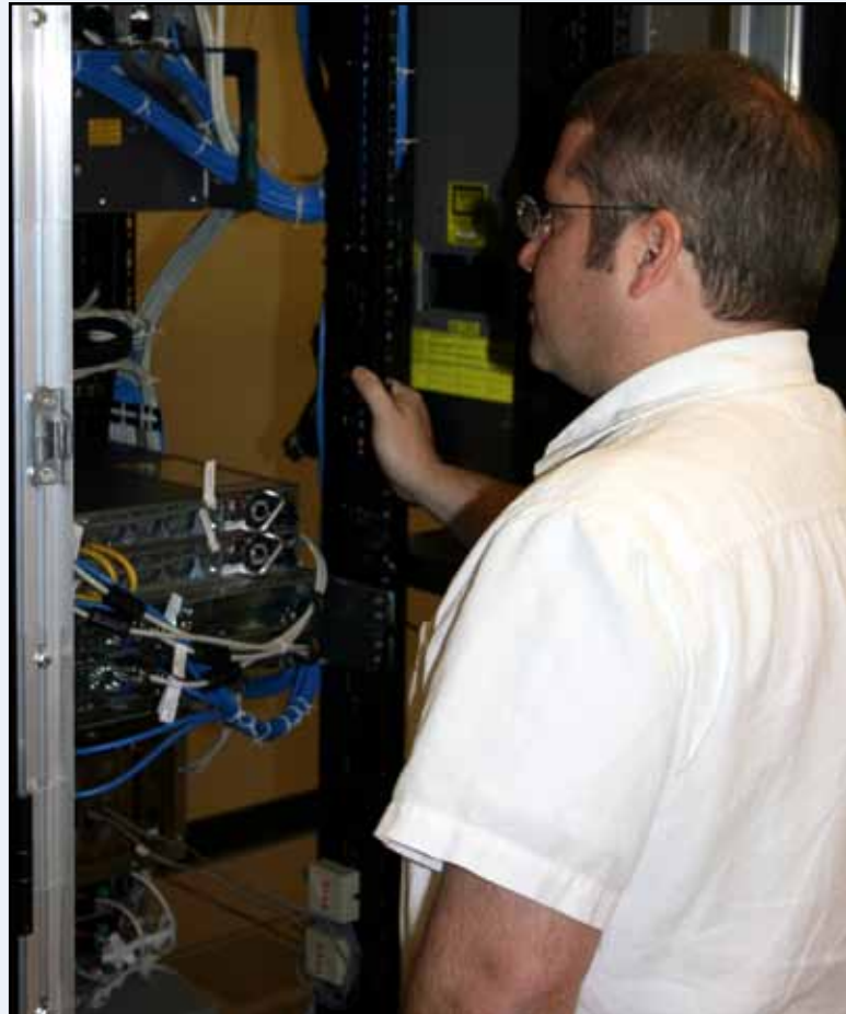
Jesse Estevez, Chariton Valley's Director of Network Operations, examines connections in the Network Operations Center (NOC). The NOC is designed to withstand tornado strength winds and provide wired phone service under the most severe weather conditions.
